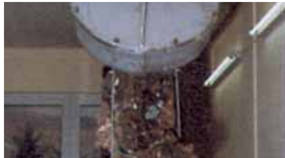
Discharge of screenings
